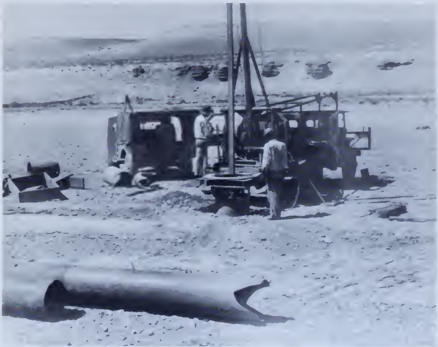
Figure 37. —Rotary digger used in exploring aggregate deposits. In the foreground is 20-inch casing, inside of which an 18-inch bucket was used for boring below ground-water level. PX-D-32042.
